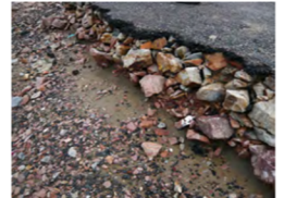
Collapsed road due to heavy trucks
