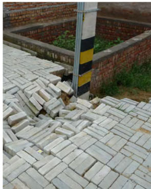
Poorly made street surfaces collapse
